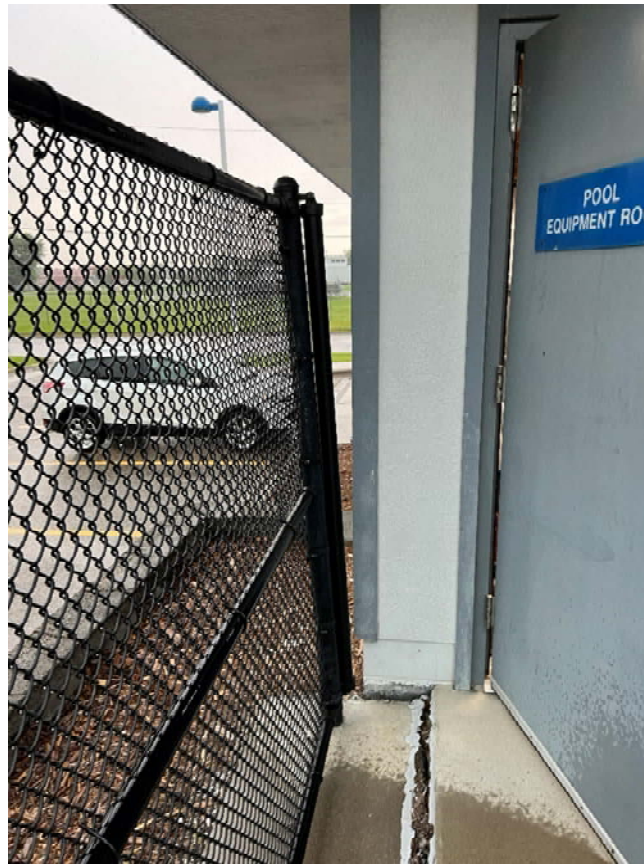
Failing Mow Strip and Fence Footings
