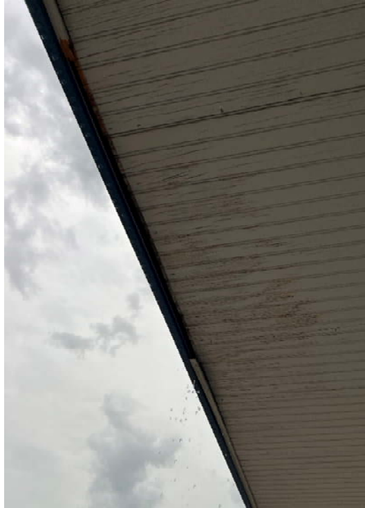
Bathhouse Eave Condition
