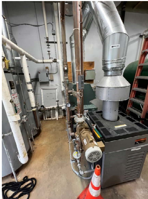
Domestic Water Heaters (Left) Pool Heaters (Right)
