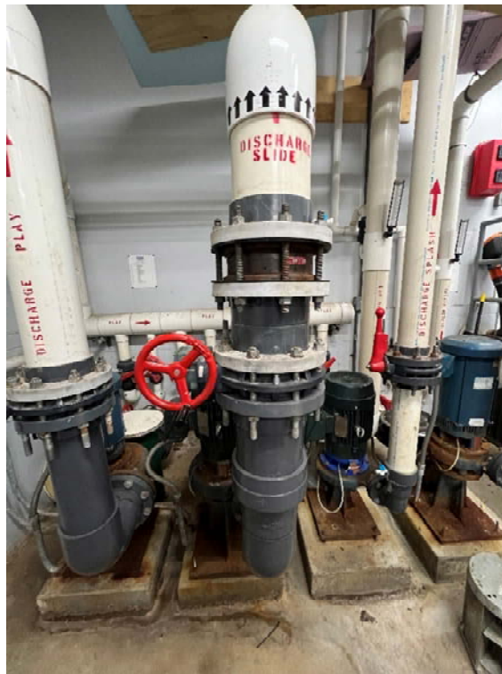
Facility Recirculation Pump Array
