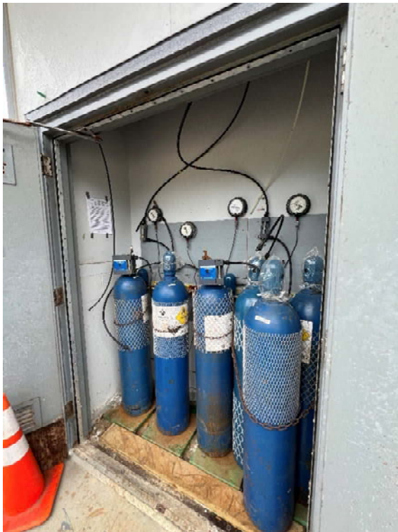
Gas Chlorine Cylinders and Storage Room
