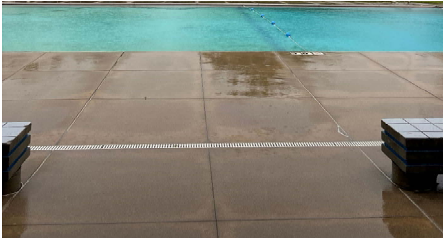
Deck Trench Drain Experiencing Flooded Condition
