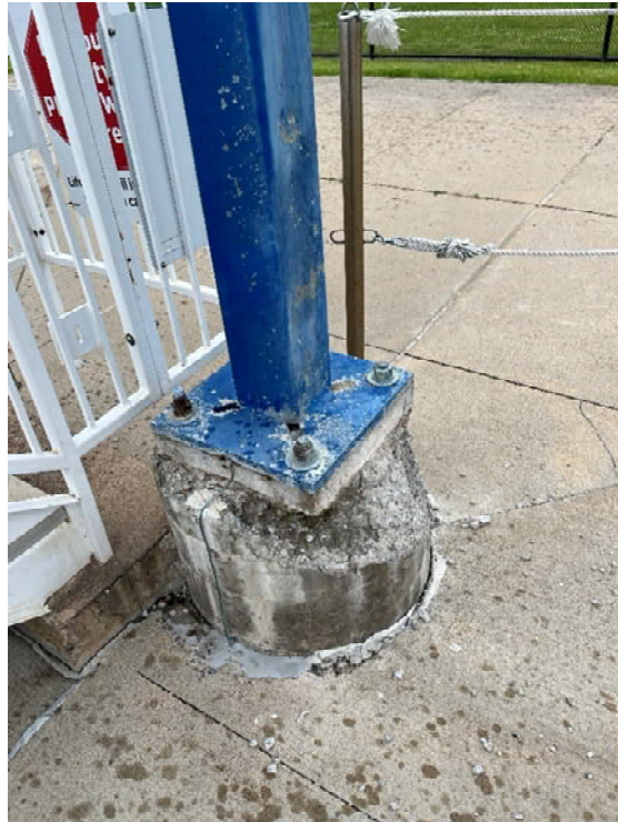
Failing Slide Foundations
